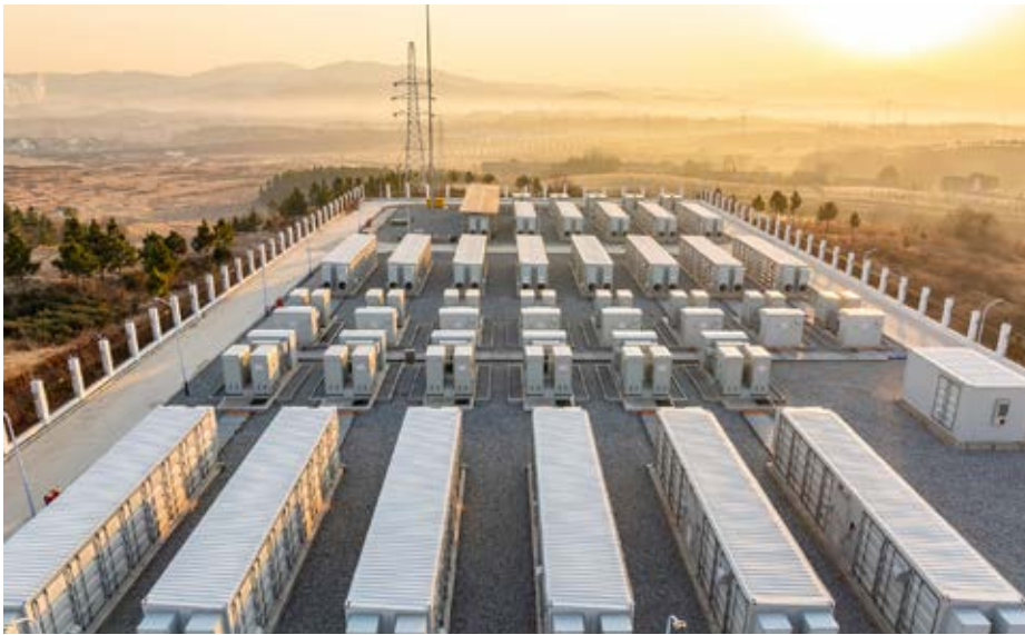
Power play Battery storage is in demand
